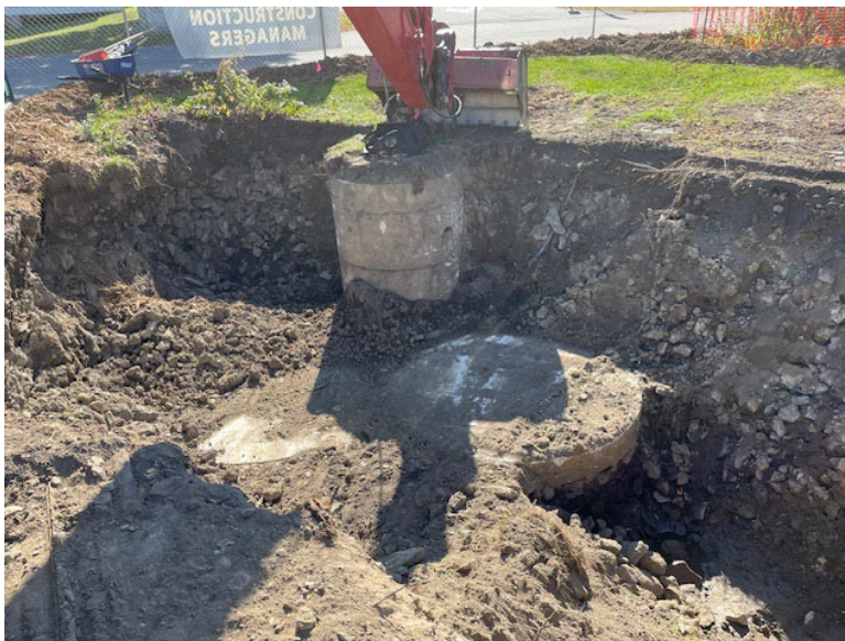
Photo above shows OT_6120 and two previously unknown grit chambers. These structures will be added to the college's stormwater map once final "as built" plans are received.
