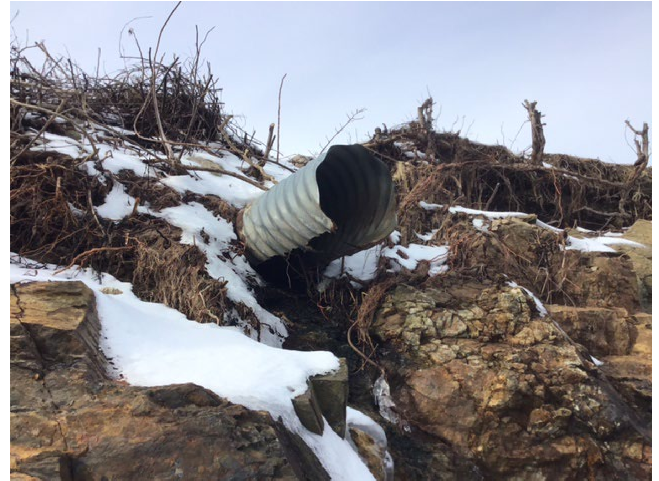
Stormwater Outfall On Willard Beach behind CSEC
